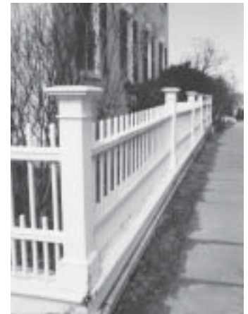
A close look at the fence around the Middlebury Community House showing the repair needs.
